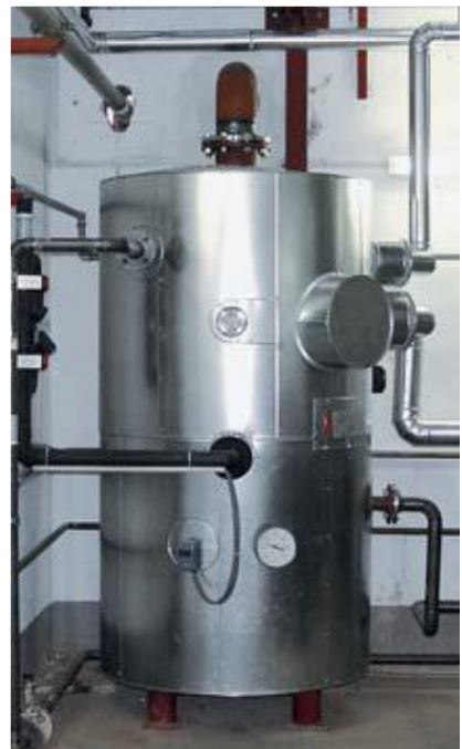
Condensate Collector Tank
