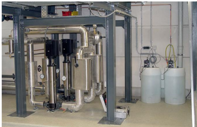
Boiler Feed Pump
